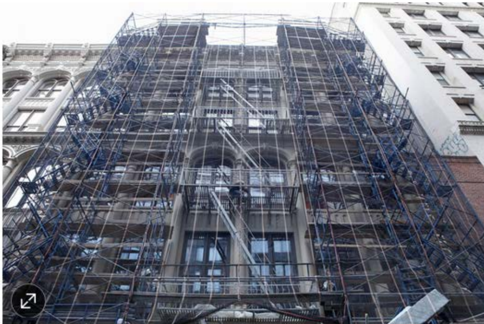
The exterior of 87 Leonard Street in New York City. ANDREW HINDERAKER FOR THE WALL STREET JOURNAL
